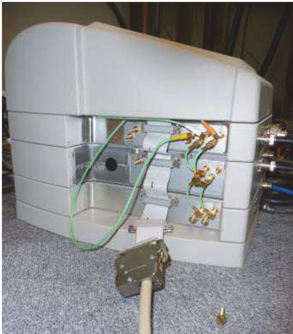
Figure 5.34: Connection of the Combiner to the Preamplifiers Flat Band Cable
