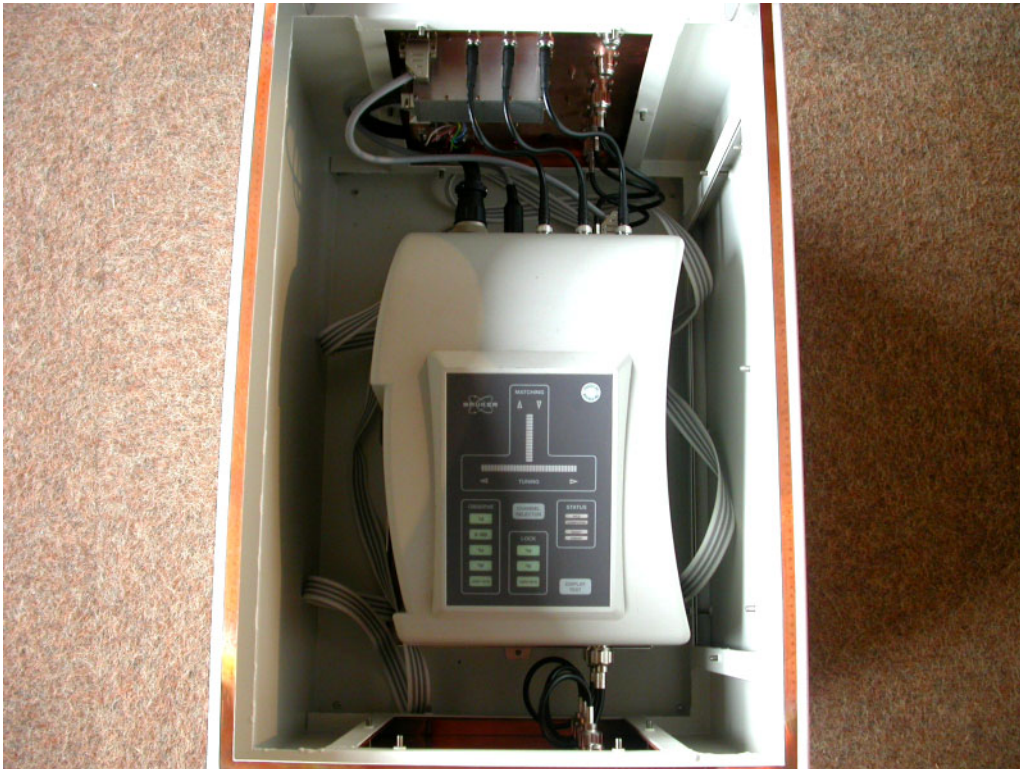
Figure 2.6. Coaxial cables connections
