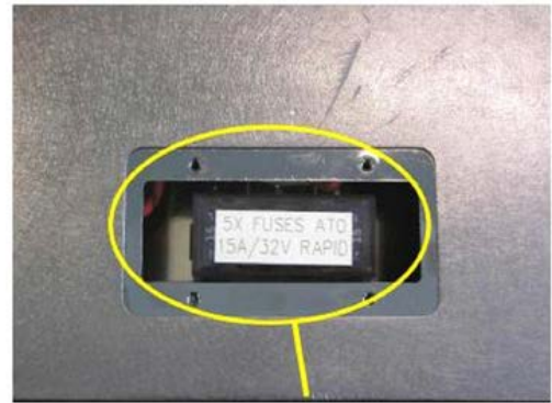
Fuse Box Cover
