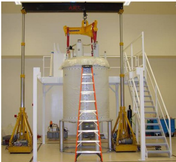
Figure 5.1: Area of Maximum Ceiling Height Needs to be Extended to Allow for the Lift System's I-beam
