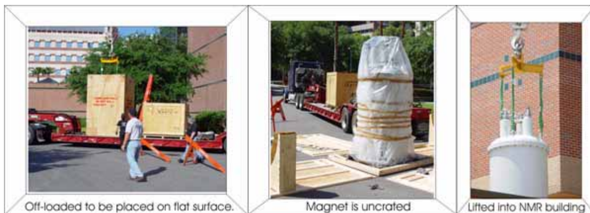
Figure 4.1. Unloading the Magnet
