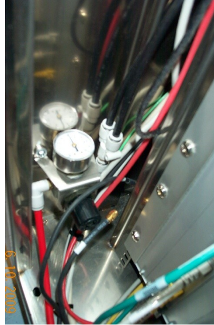
Air regulator and gauge in Single bay
